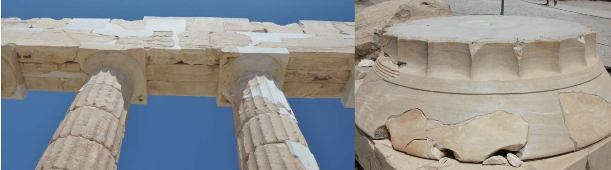
Fig.2: The columns of the Parthenon (left) employ a dry-assembly, interlocking system where wooden pins are placed in the central alcove of each drum (right) to align the structure. Overall stability is ensured by the own weight of the structure.
