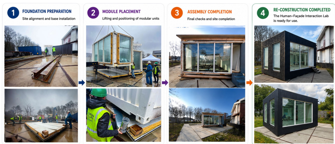
Fig. 2: The process of re-assembly: 1. Preparation of the foundation; 2. Module placement; 3. Assembly completion and start of re-construction and upgrading work; 4. Reconstruction according to the new design and capabilities.
