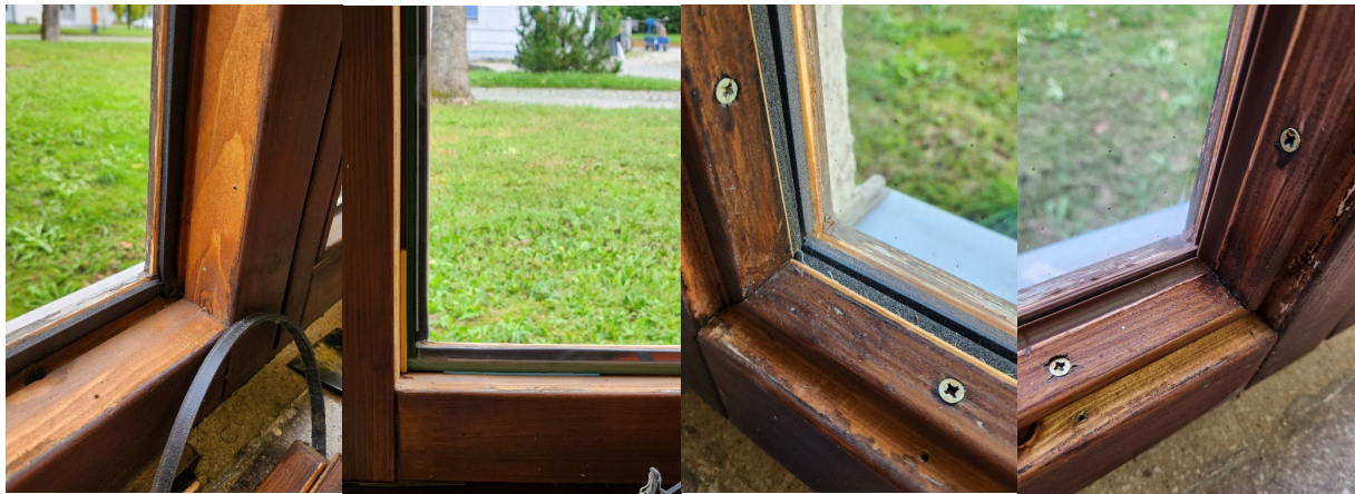
Fig. 4: Detail of corner from inside in different installation steps: window frame with attached new foam strip at glazing rebate upstand, VIG in position with setting blocks, glazing bead with attached new foam fixed with screws, seal attached.
