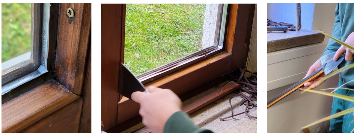
Fig. 3: Dismounting steps (left to right): corner detail before dismounting IGU, after cutting seal and removing screws glazing bead are removed using spatula, glazing bead is cleaned from old foam by using putty knife.
