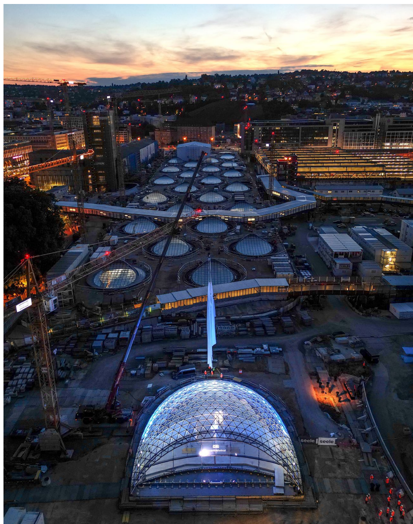
Fig. 12: Opening of the Grid Shell Staatsgalerie with the Light Eyes behind ©DB Projekt Stuttgart–Ulm.
