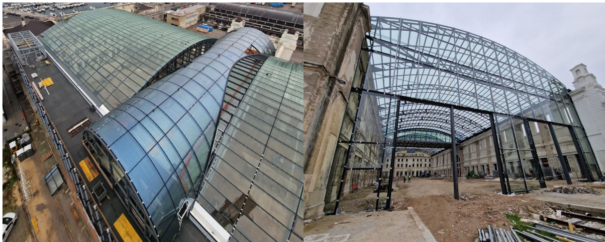
Fig. 10: Exterior views of the roof and of the main glazed façade during construction.
