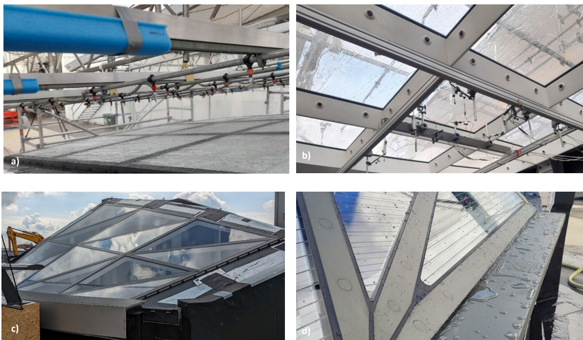
Fig. 9: Performance mock-up of the gridshell: a) view from outside with spraying system b) view from inside c) overview of mock-up d) water tightness test © seele.
