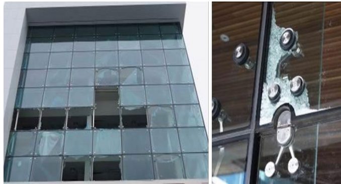
Fig. 2: Seismic damage to PFGFSs (Baird et al., 2011).
