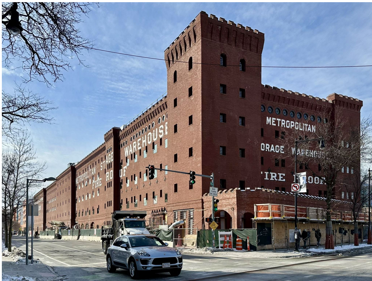
Fig. 1: Metropolitan Warehouse during renovation, viewed from the southeast corner of the building.
