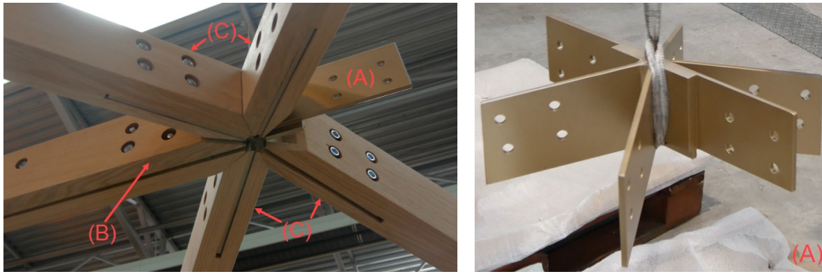
Fig. 6: Detail of different connection during the pre-assembly. (A) 6-point steel “star”. (B) Steel-to-steel connection. (C) Timber-to-steel connection.
