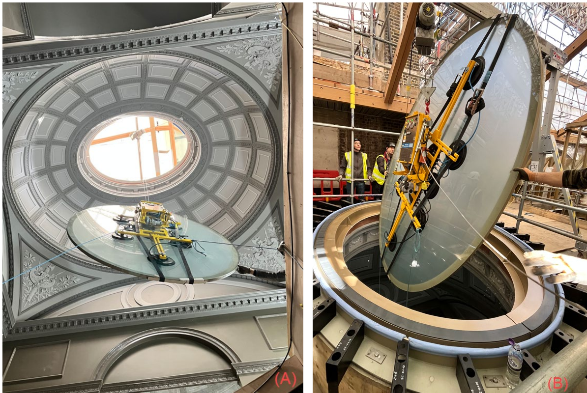
Fig. 12: Oculus. (A) Lifting of the glass panel from the floor below. (B) Installation of the glass panels.
