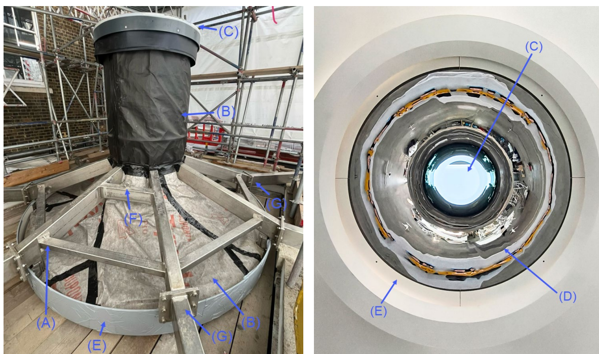
Fig. 9: Terrace rooflight. (A) Supporting structure. (B) Mineral wool insulation. (C) DGU. (D) Inverted funnel. (E) Support plates for the chandeliers. (F) Lifting eye. (G) Detachable supports.
