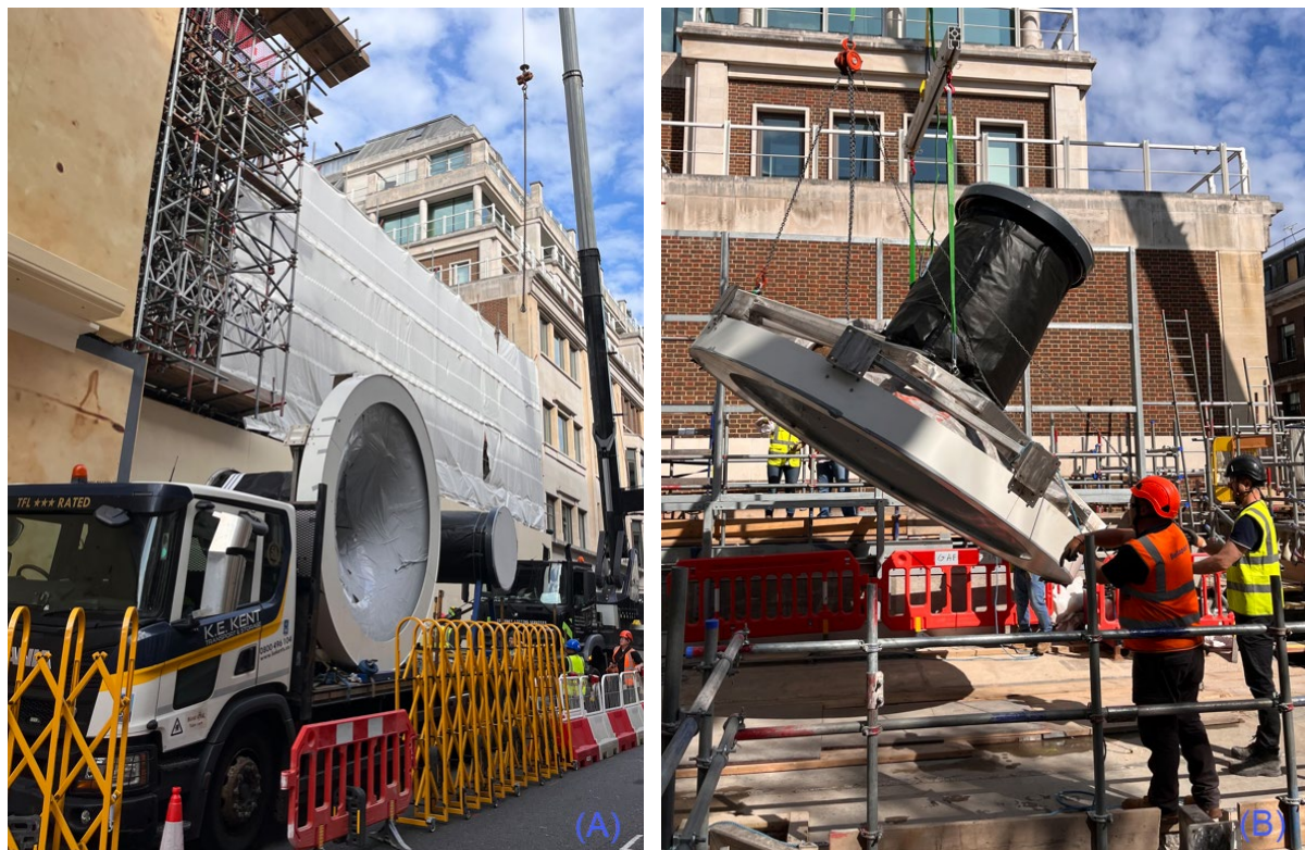
Fig. 10: Transport and installation of the terrace rooflights. (A) Transportation of the pre-assembled units. (B) Lifting and turning the pre-assembled rooflight on site.
