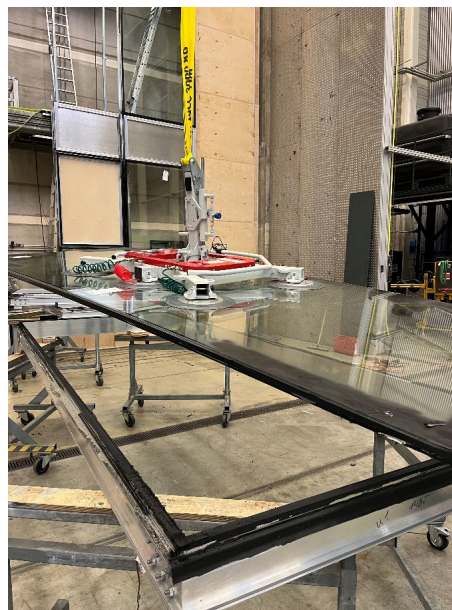
Fig. 20: Suction cups used to remove the glass pane from the aluminium frame.
