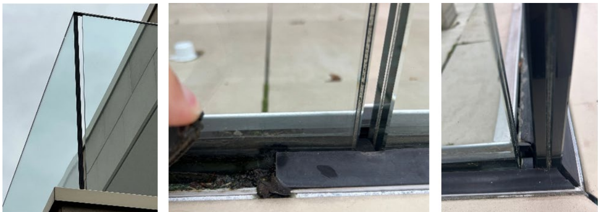
Fig. 4: Moisture and freeze–thaw effects affecting elastomers and positional stability.
