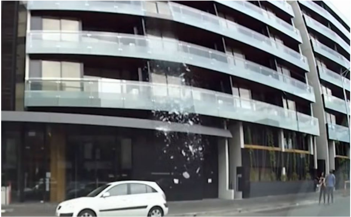
Fig. 2: Spontaneous fracture of balustrade.
