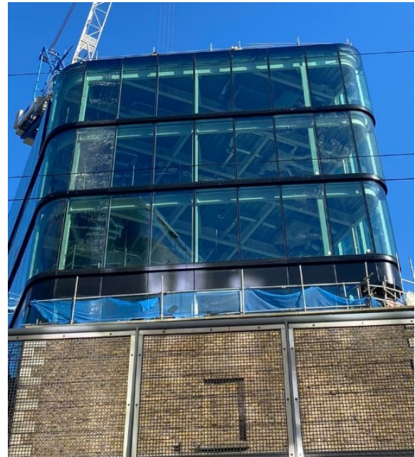
Fig. 3: The Malthouse, Dublin - curved SSG (GLF Facades).
