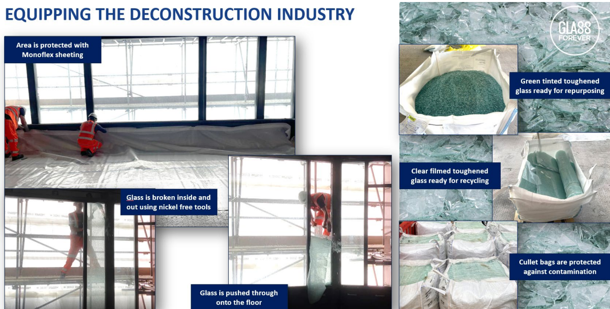
Fig. 6: An example of how the deconstruction of a façade was modified to recover the glass.
