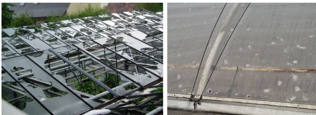
Fig. 2: Hail damage at greenhouses (Österreichische Hagelversicherung VVAG - Austrian Hail Insurance Agency).
