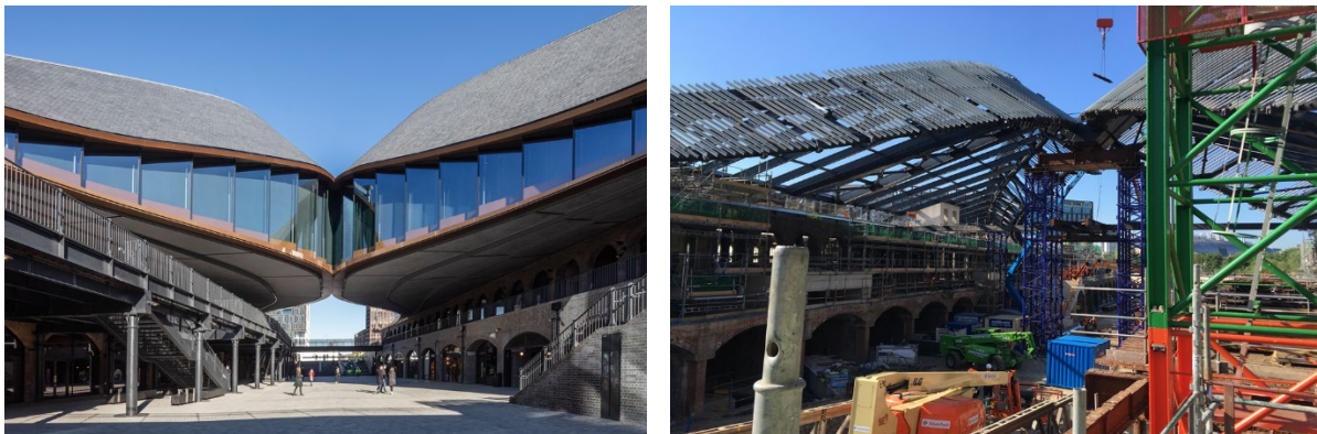
Fig. 10: Left - Finished façade, Right – Project during the construction of the primary structure
