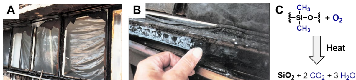
Fig. 1: Example of bonded glass units after exposure to a real external fire: the glass shards are still retained on the aluminum frame (A) and the silicone shows a char on its surface (B). The char formation follows an oxidative process resulting in silicate-like (SiO 2 ) structures (C).
