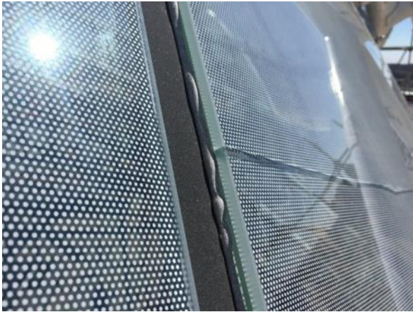
Fig. 7 Thermal crack in panel.
