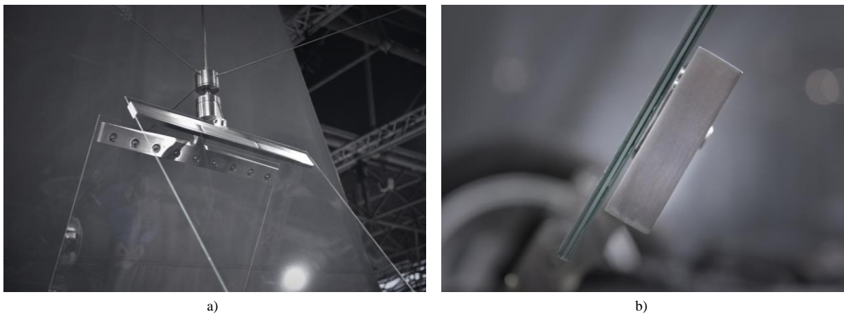
Fig. 12 a) Pivot detail with frictionless rotation and swinging ability, b) One-sided eccentric bracket detail (© DefineEngineers / Carpenter | Lowings / seele).
