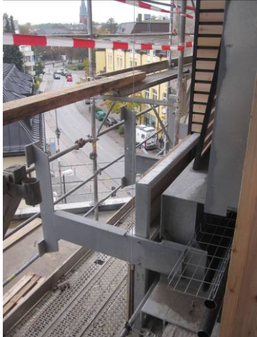
Figure 4: Installed Steel Fin.
