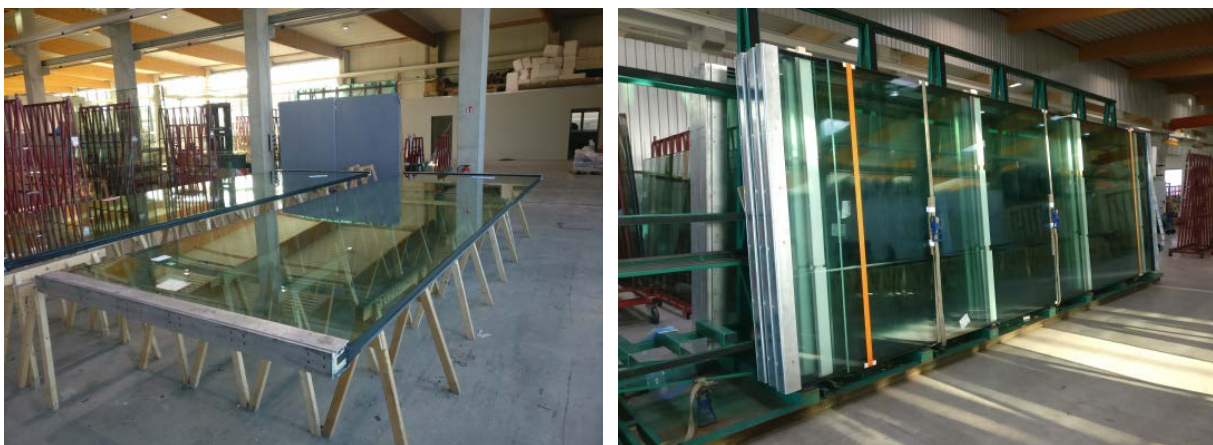
Fig. 5 Manufacturing of the insulating glazing and assembly of the metal profiles in the Thiele Glas plant, Wermisdorf. Delivery on a glass rack to the construction site with an in-loader.
