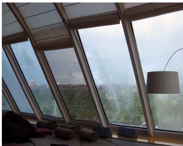
Fig. 2 Insulating glass units with moisture in the closed cavity between the glass panes
