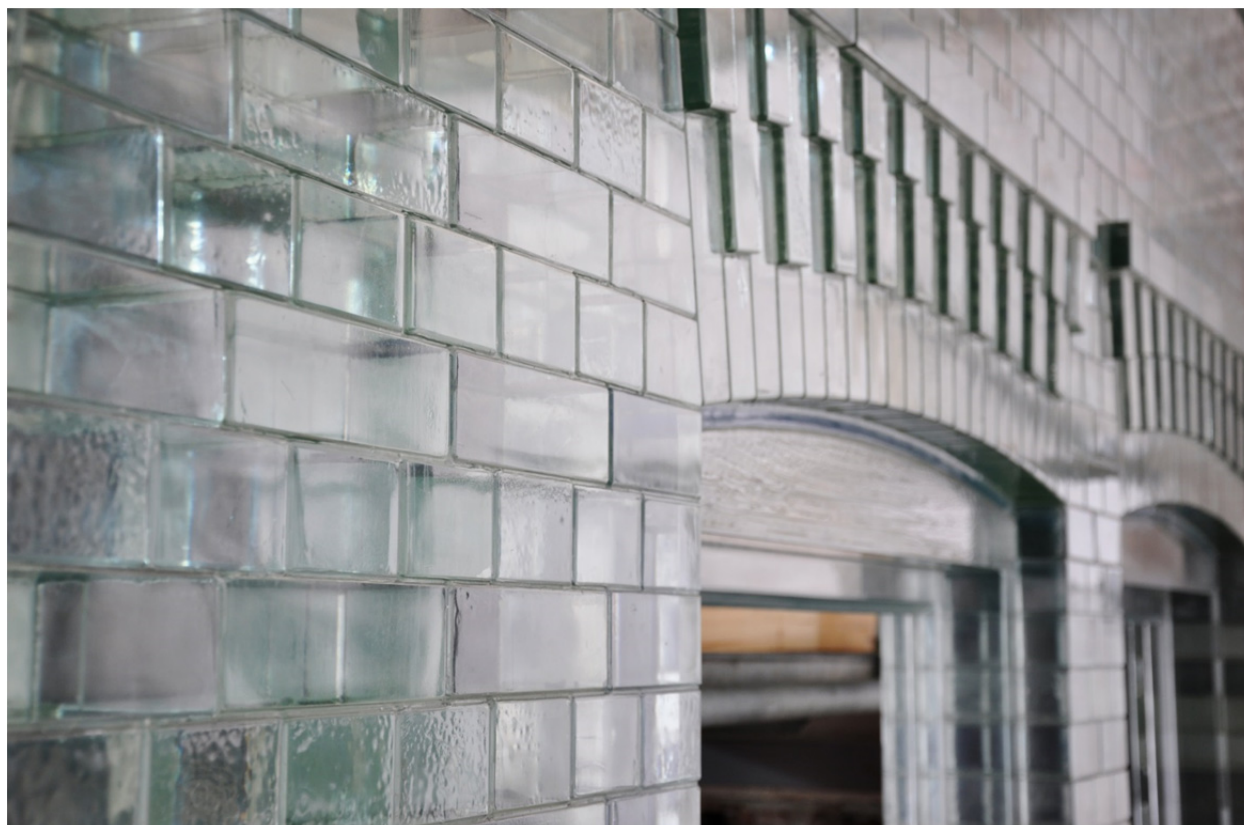
Fig. 14 Close up of glass masonry wall, the architraves and the cast glass window frames.
