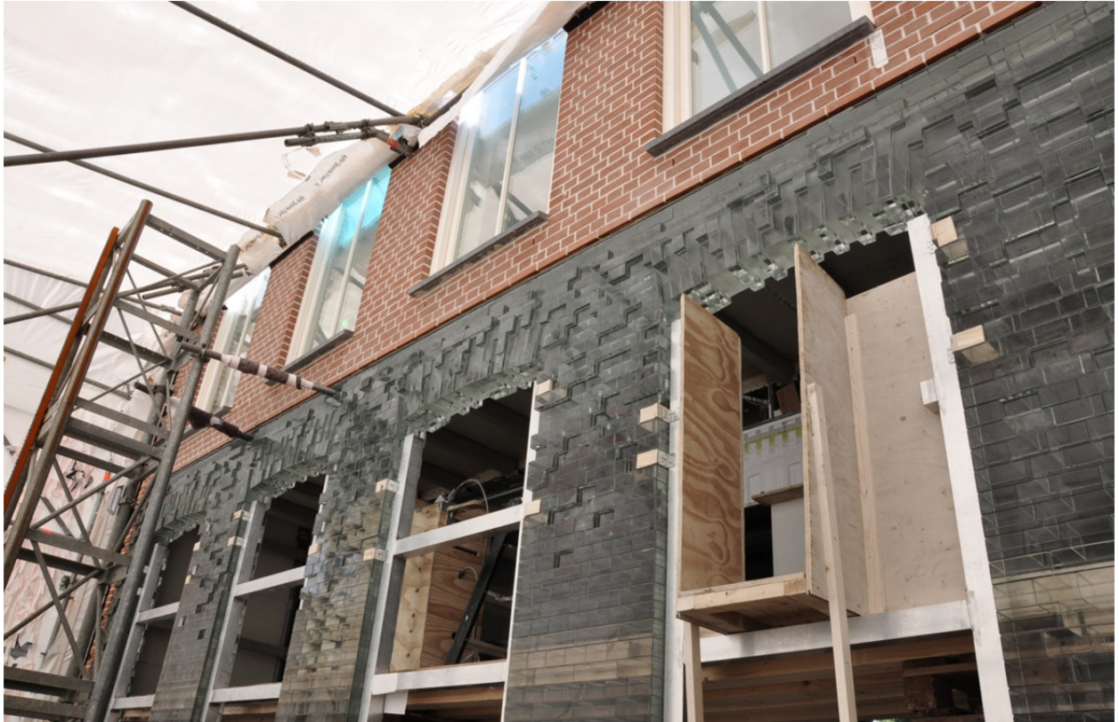
Fig. 9 Completed glass brick wall with the 40 mm narrower bricks bonded on location.
