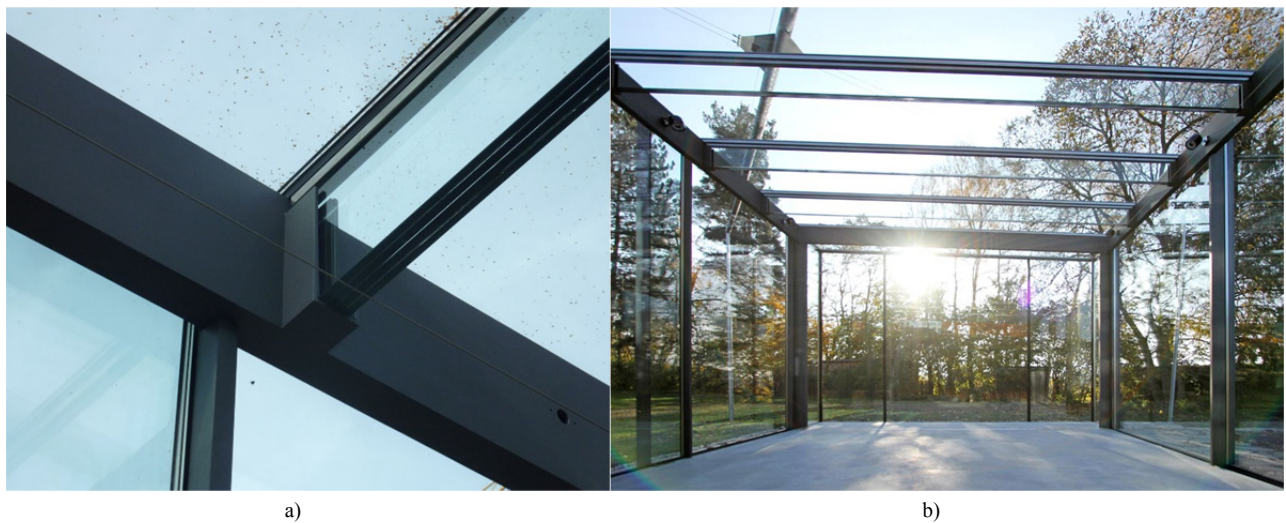
Fig. 5a) and b) Glass fin with socket detail and view from inside ( www.master-ateliers.com ).
