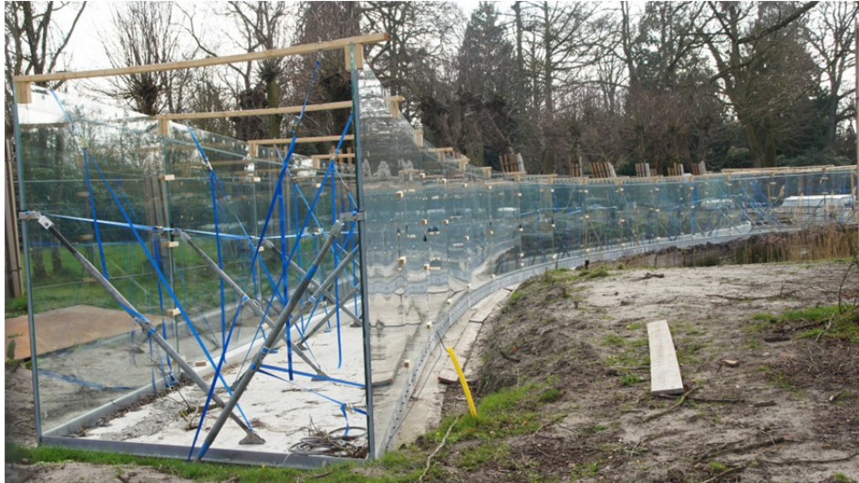
Fig. 15 End of wing, under construction, visible is the clamping in the foundation.
